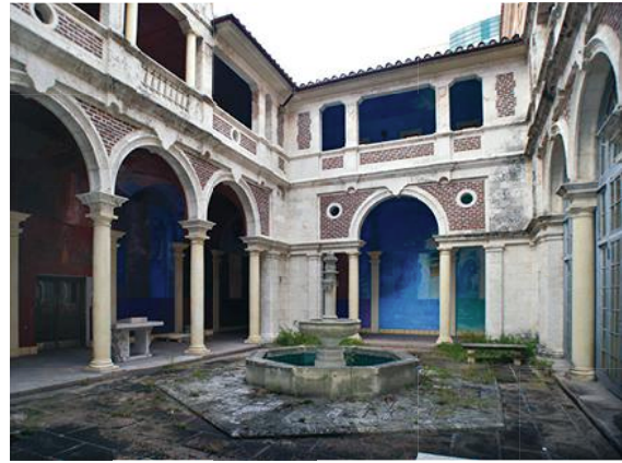
(Before) The inner courtyard of Dyer courthouse will be enclosed and transformed into event space for students in Miami Dade College's School of Design, Engineering and Technology. Photo: LEO A DALY
