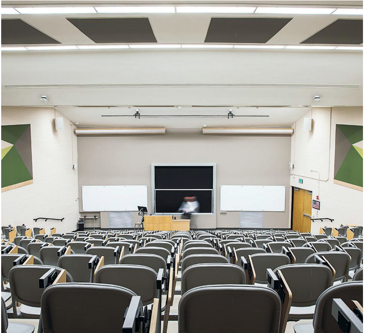
The Audacy System is installed in an auditorium in the Engineering Building at Colorado State University.
